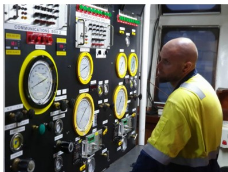
DEEPWORX SATURATION CHAMBER CONTROL RUN BY THE LSS AND LST
